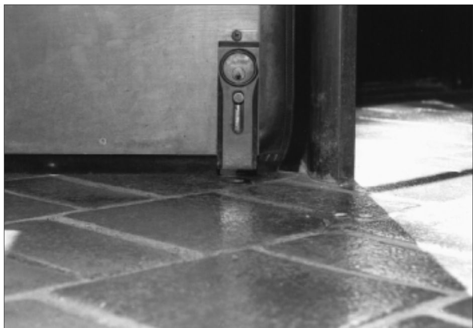
3. Although a new, raised floor would have been preferable, the lowered door lock was the best solution for this customer's revolving door lock problem.
