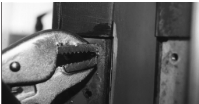
4. After drilling plenty of screw was left to grasp with a vise grip. This screw was easily removed after first soaking it with a rust penetrant.
