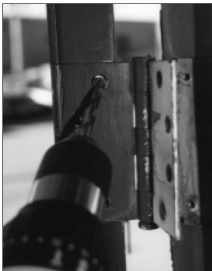
3. Screws that are corroded and uncooperative may need to be drilled. Using a Black & Decker Bullet Point bit makes this job fast and easy.
