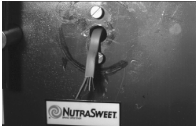
5. The cable has been cut before attaching male 8-pin connector.
