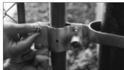
3. Place the push button lock up to the gate and fasten with the four carriage bolts.
